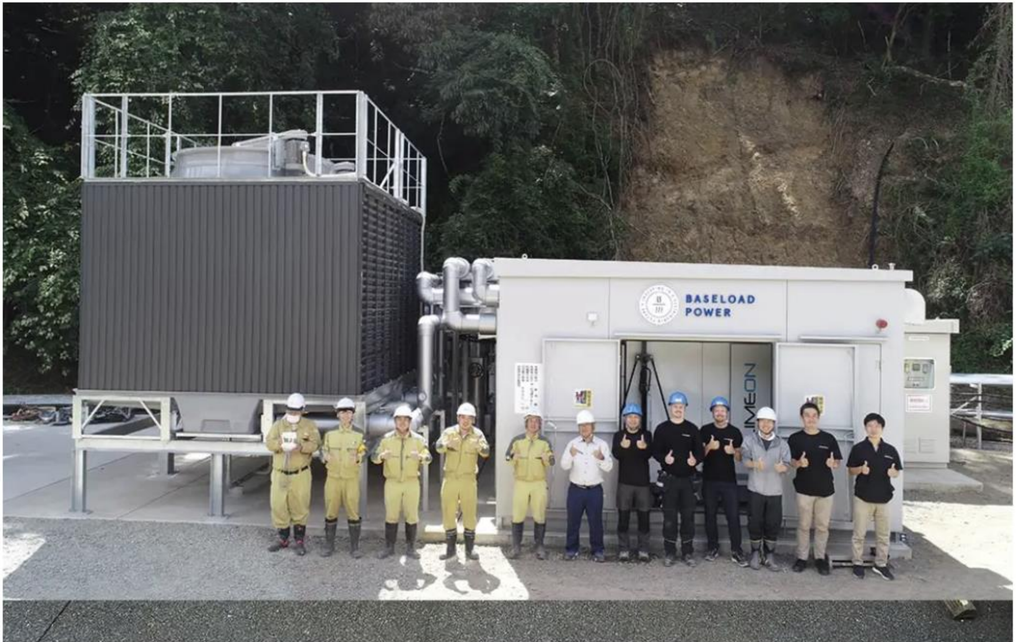
Small Scale (2MW) Geothermal Facility
