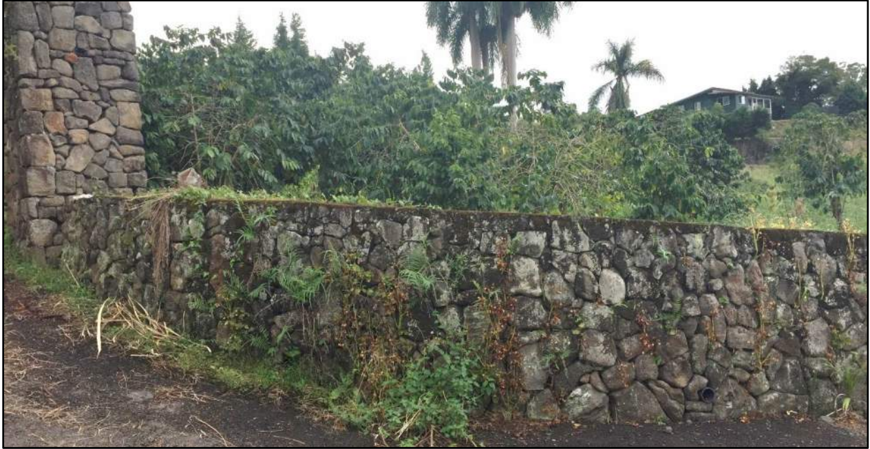
Figure 24. Photo showing the southern portion of the modern stone wall fronting the project area along Māmalahoa Highway; note PVC drainpipes along the base of the wall; view to southeast
