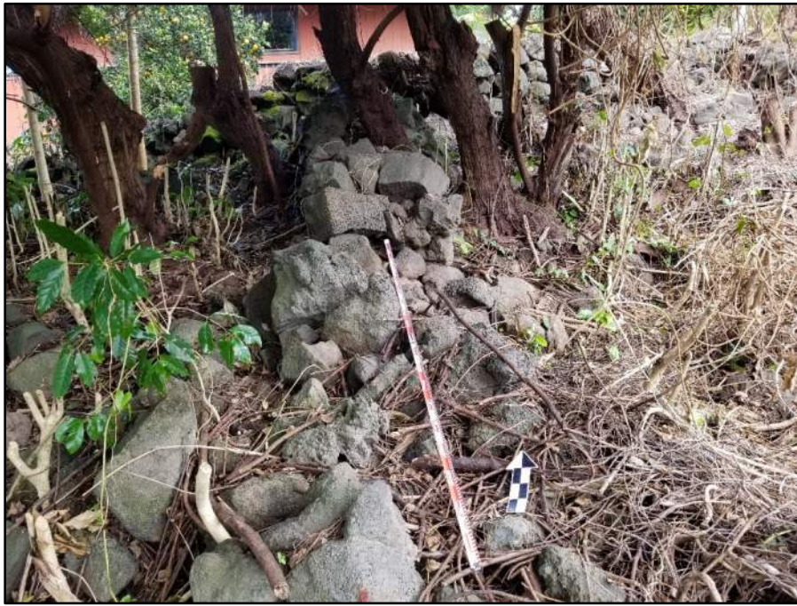
Figure 102. Photo showing the southern impacted portion of SIHP # -31124 Feature B terrace wall; view to north
