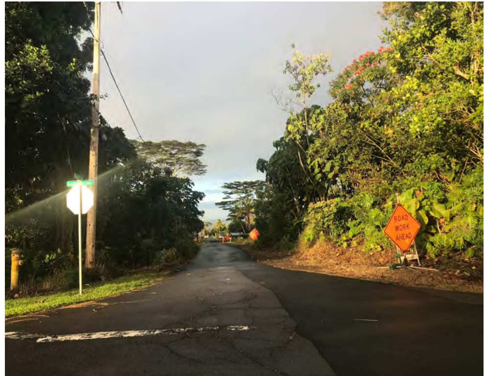
Sewerline installed but not turned over to County until we resolve MOA and fees.
