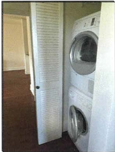
In unit stack laundry
