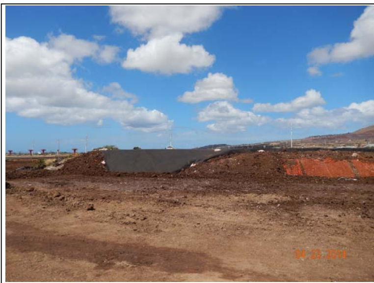
Photograph 18: View of fill area with geomembrane liner and orange construction fence visual indicator.
