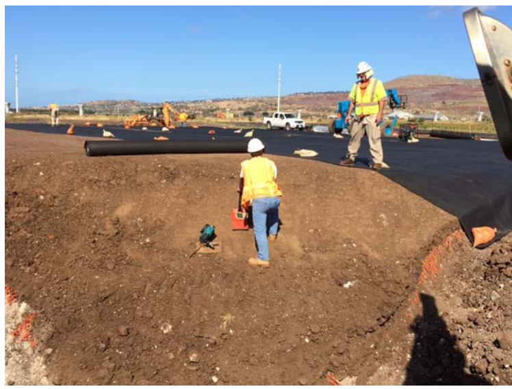
Photograph 13: Hirata & Associates checking soil compaction prior to placement of fabric and liner.
