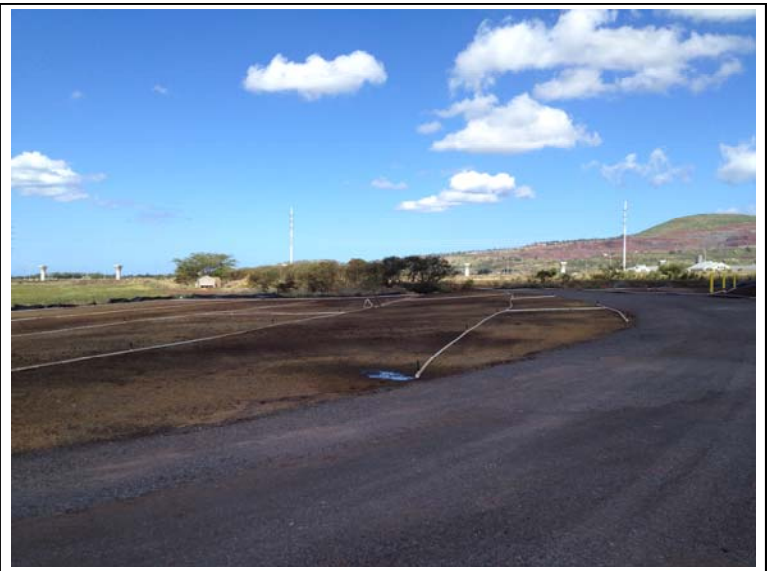
Photograph 32: View of former excavation area and haul road. Hydroseeding complete, granular material used to fill haul road.
