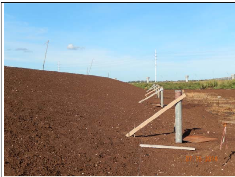
Photograph 30: View of pipe bollards prior to filling with concrete, installed along the perimeter of the capped area.
