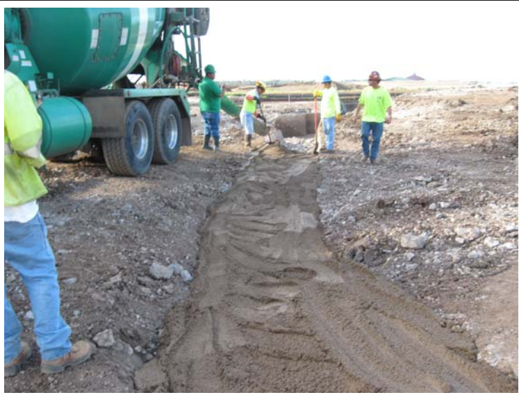
Photograph 7: CLSM used to fill irrigation ditch after demolition of concrete culverts beneath haul roads.
