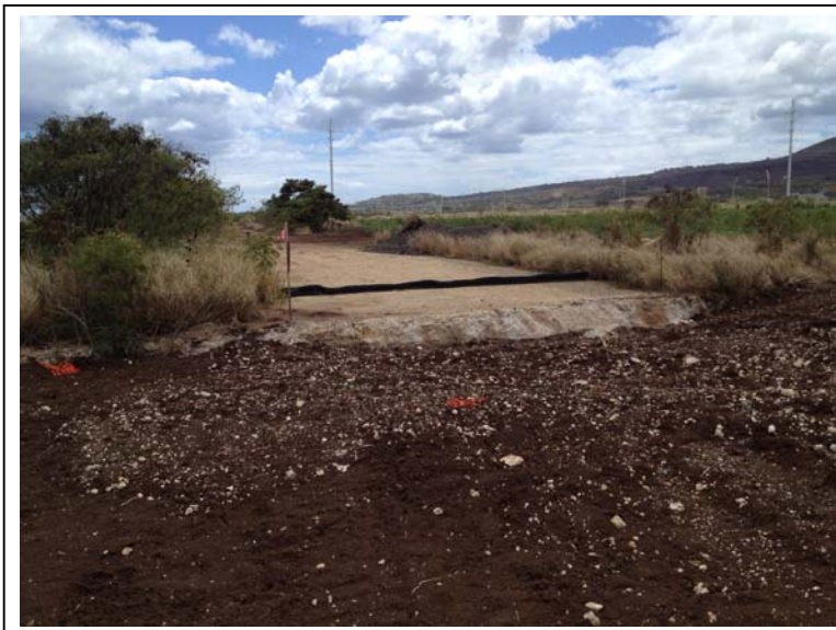
Photograph 27: View of backfill material near haul road prior to placement of imported granular fill.
