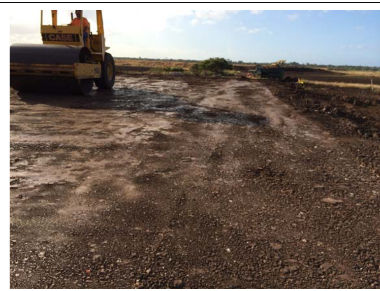
Photograph 12: Compacting low permeability soil prior to placement of geotextile fabric and geomembrane liner.
