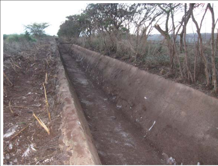
Photograph 4: Soil from concrete-lined irrigation ditch removed and placed within PML site. No breaks in concrete-lined ditch observed.
