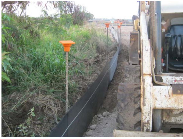
Photograph 1: Silt fence and other storm water BMPs installed prior to start of construction.
