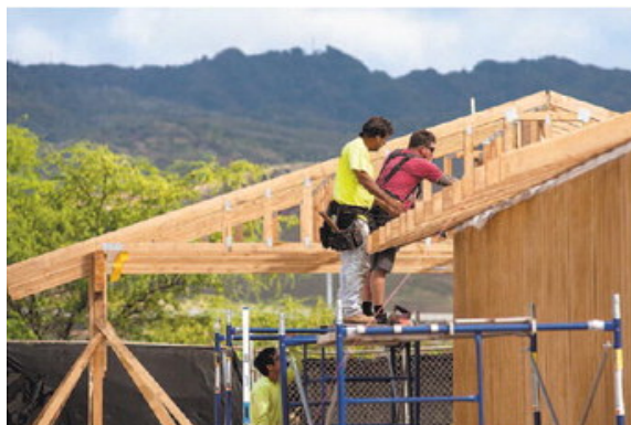
Builders worked on the roof trusses of a home in Kapolei on Thursday, one of several being built on vacant lots in the Kauluokahai homesteading subdivision.
