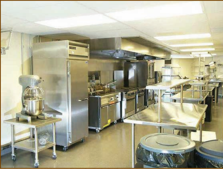
Sample Commercial Kitchen
