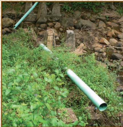
Broken Irrigation Pipe
